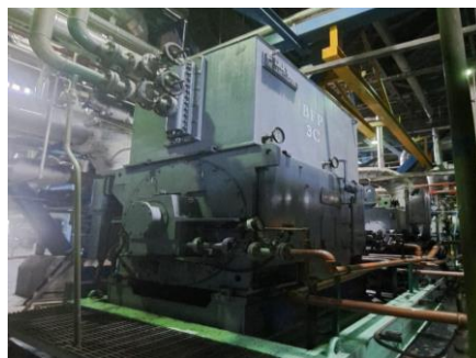
Gambar 2 Motor Induksi Tiga Fasa Boiler Feed Pump
